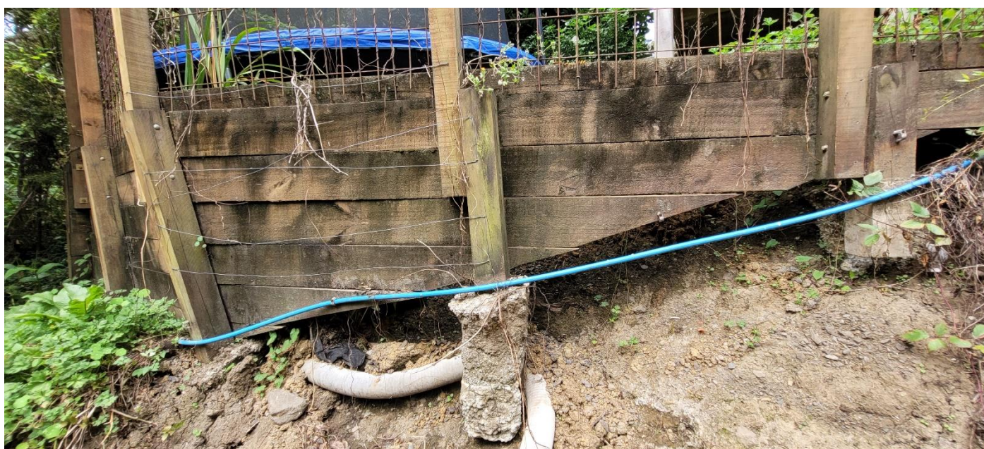
Photo 4: Undermined section of RTW-02, looking south.
